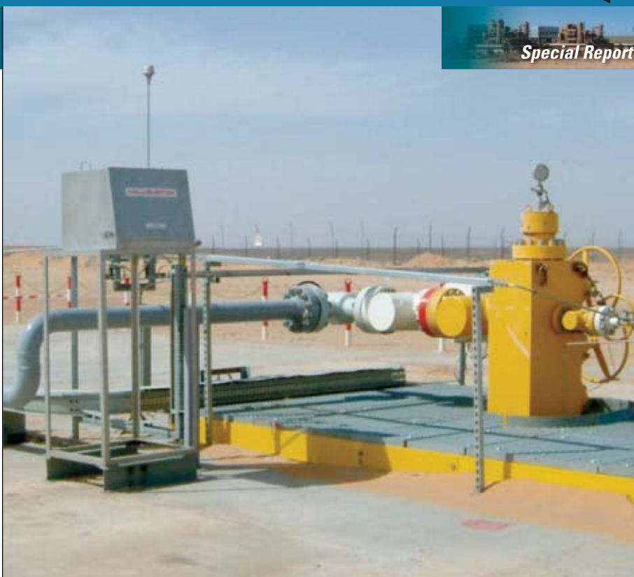
Carbon dioxide injection wells are part of Krechba, one of eight Algerian gas fields that are part of the In Salah gas project. Operators inject CO 2 into a deep saline formation. Photo from BP PLC.
